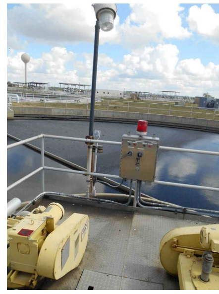
PRIMARY CLARIFIER NO.2 PHOTOGRAPH B
