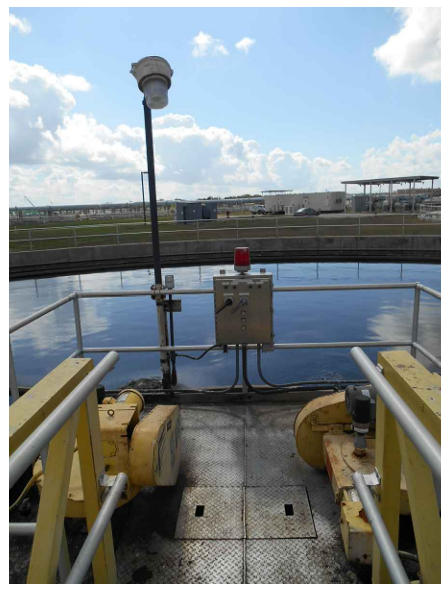
PRIMARY CLARIFIER NO.8 PHOTOGRAPH B
